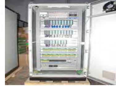
DCS & Transmission Systems
